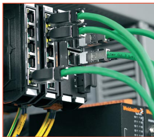
INDUSTRIAL ETHERNET, SWITCHES AND CABLING
